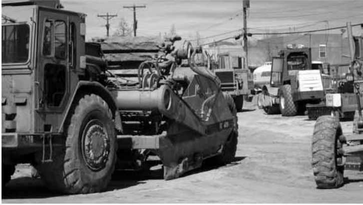
- Construction machinery stands ready to begin work at Plaza Feliz, a 65-unit apartment complex being built in Albuquerque's Trumbull Village.
