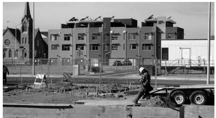
- Construction begins on Silver Gardens II, an affordable apartment community in Downtown Albuquerque.
